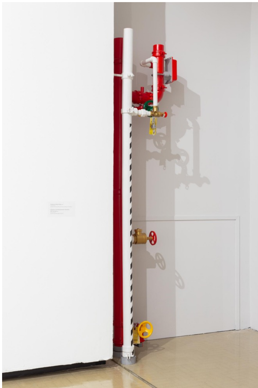
«Whitney Fire Suppression System (between Calder and Oiticica)» tall red pipes, 2022
